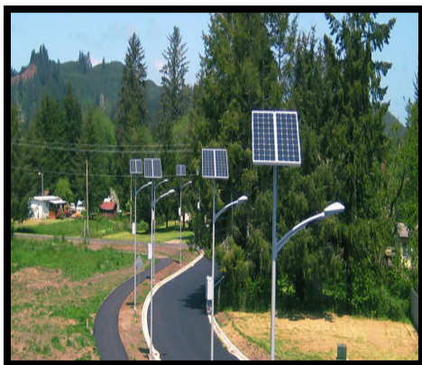
9.6 Solar street light
